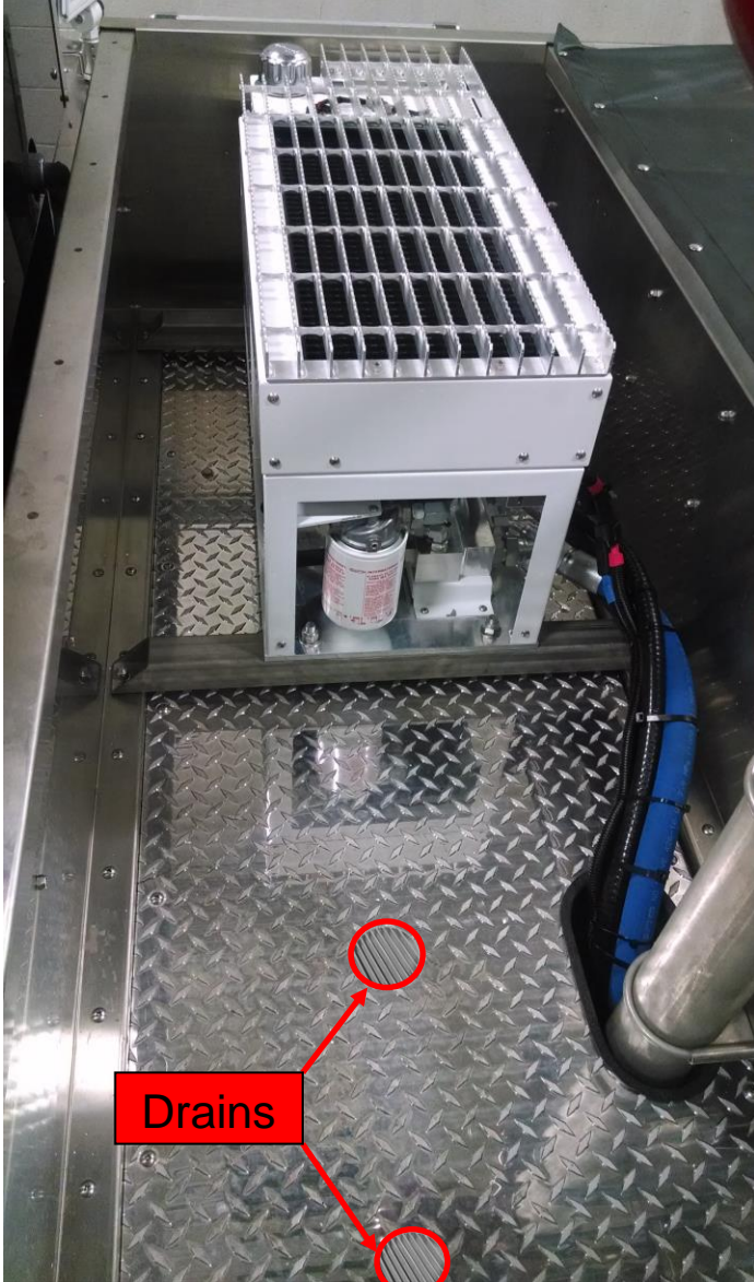
GOOD Installation/Proper Drainage
