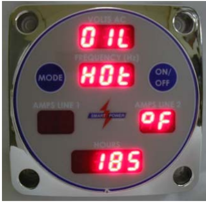
Figure 5: Command and Control Center Overtemperature Readout
